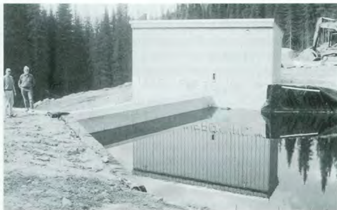
Celsius. The head pond can store water during interruptions to the circuit, preventing lost revenue due to spill during outages.
