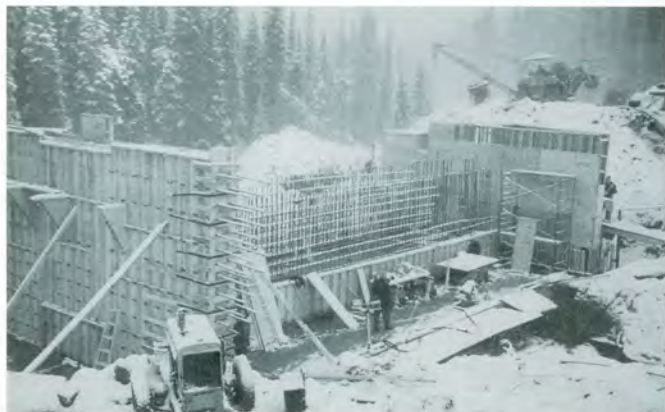
Construction of the intake for 7-MW Hystad Creek was completed during the winter, when temperatures fell as low as minus 30 degrees
