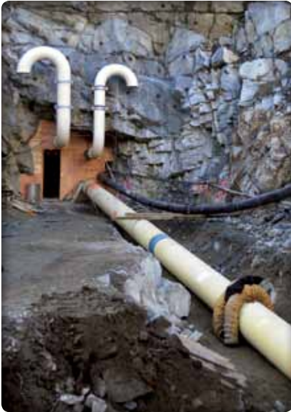
Pictured is the lower end of the tunnel during construction. In addition to the main penstock, a smaller return pipe is used to pump water back up to the source of Tyson Creek to maintain constant flow in the creek bed. The curved white pipes vent the tunnel.
