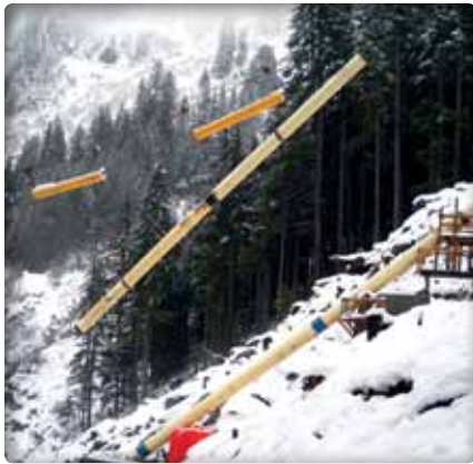
A suspended cable "skyline" moves a 26-meter penstock section into position on a grade too steep for conventional machinery.
