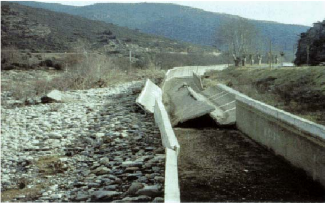
Photo 4-12 Channel destroyed by uplift pressure
