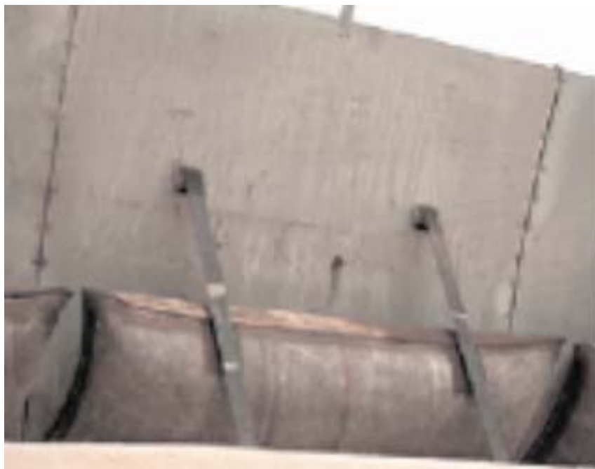
Photo 5.6: Flashboard controlled by inflatable rubber bladder
