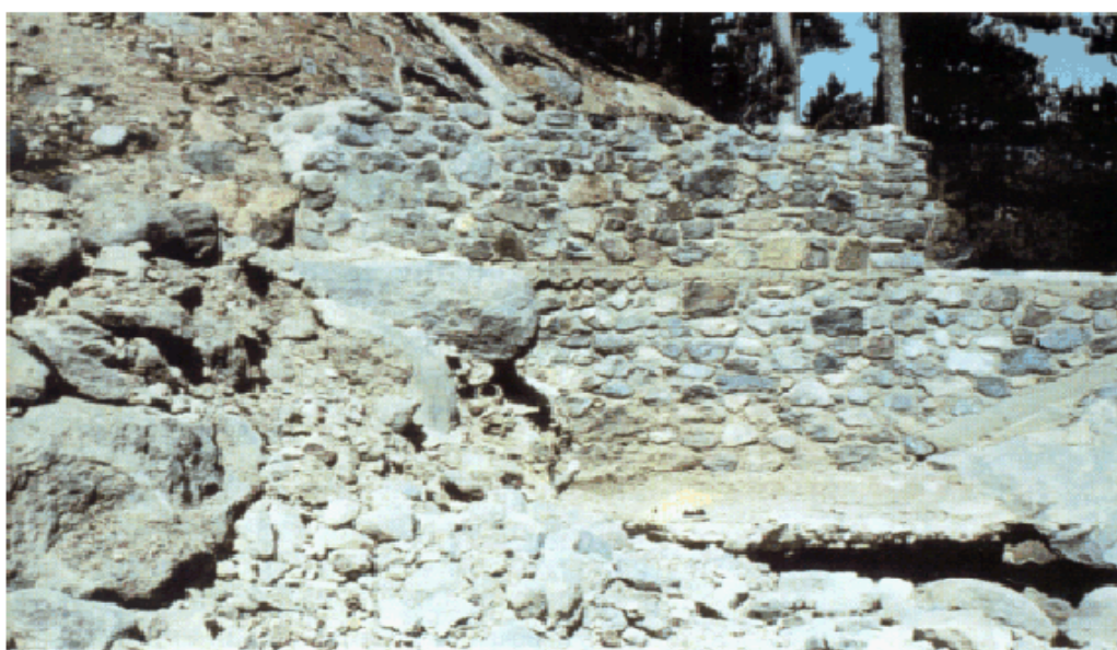
Photo 4-11 Weir undermined by seepage
