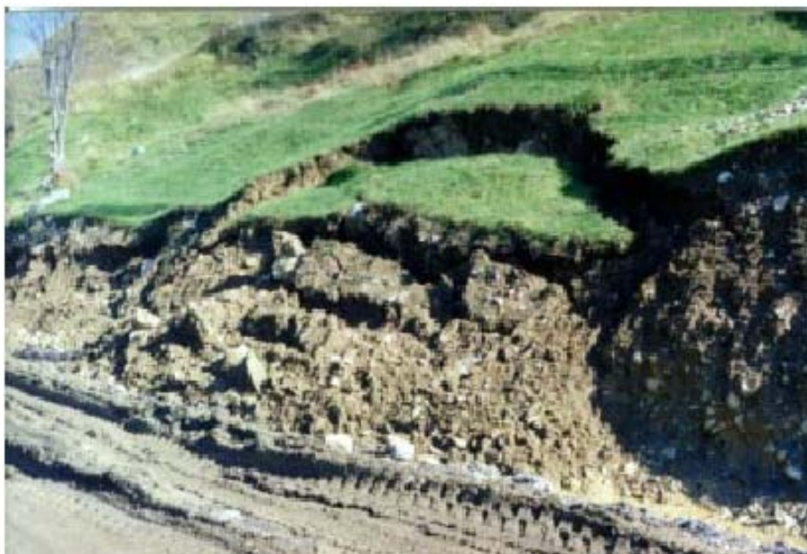
Photo 4-2 Local instabilities generated during the excavation works
